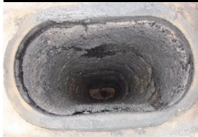
Thick Creosote Buildup in Chimney
